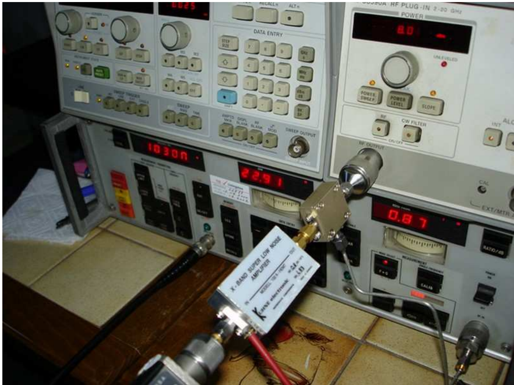
F5DQK February 2009 part 2/4 2 to 18 GHz NF+gain measuring with Eaton 2075 or HP 8970b and ADDS
